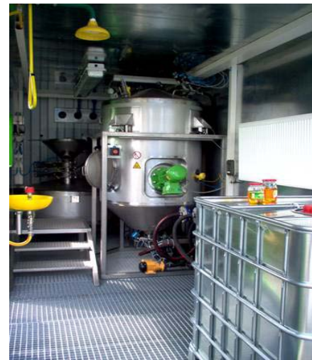
Inside view of biodiesel system (900 t/a)
