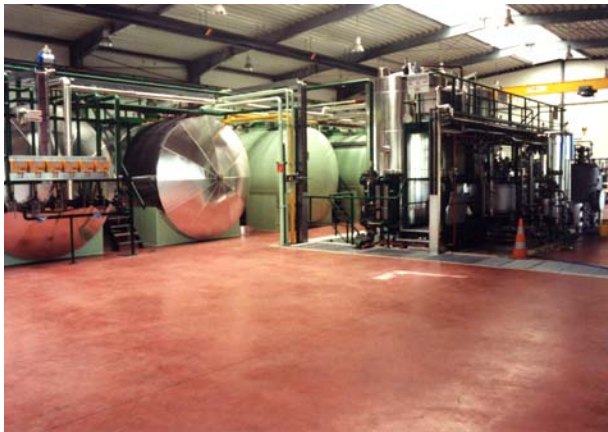
Biodiesel plant in Germany (5,000 t/a capacity)
