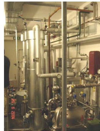
Inside view of biodiesel system (5,000 t/a)
